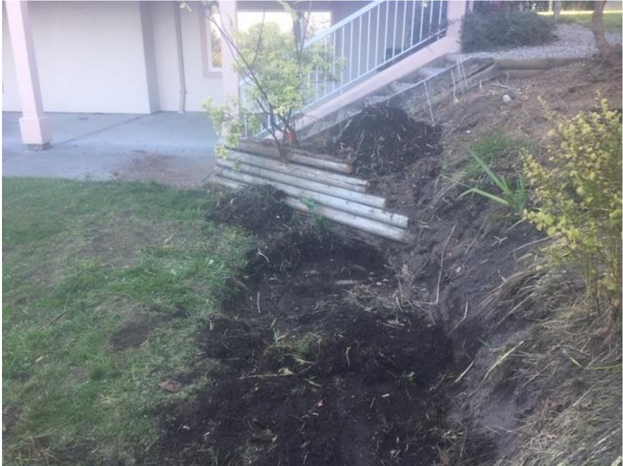
2 nd septic tank (bottom of the house comes here)
