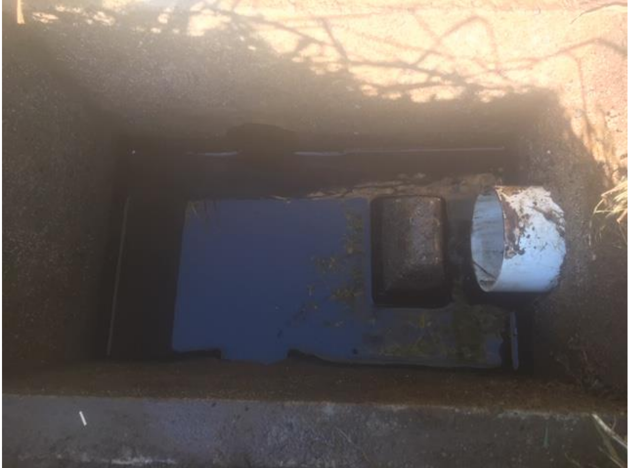
Same box after the cleaning
