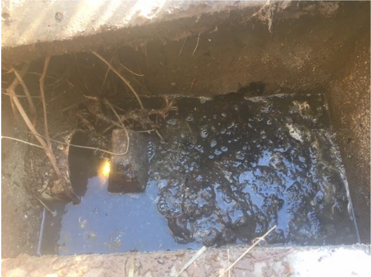
Distribution box (lower field); this photo was before the field got cleaned
