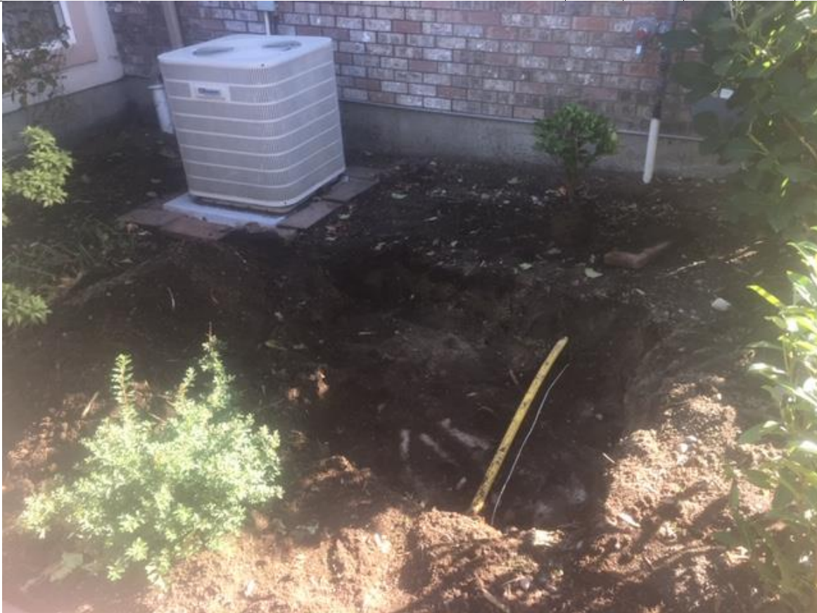
Location of 1 st septic tank ( top part of the house comes here)
